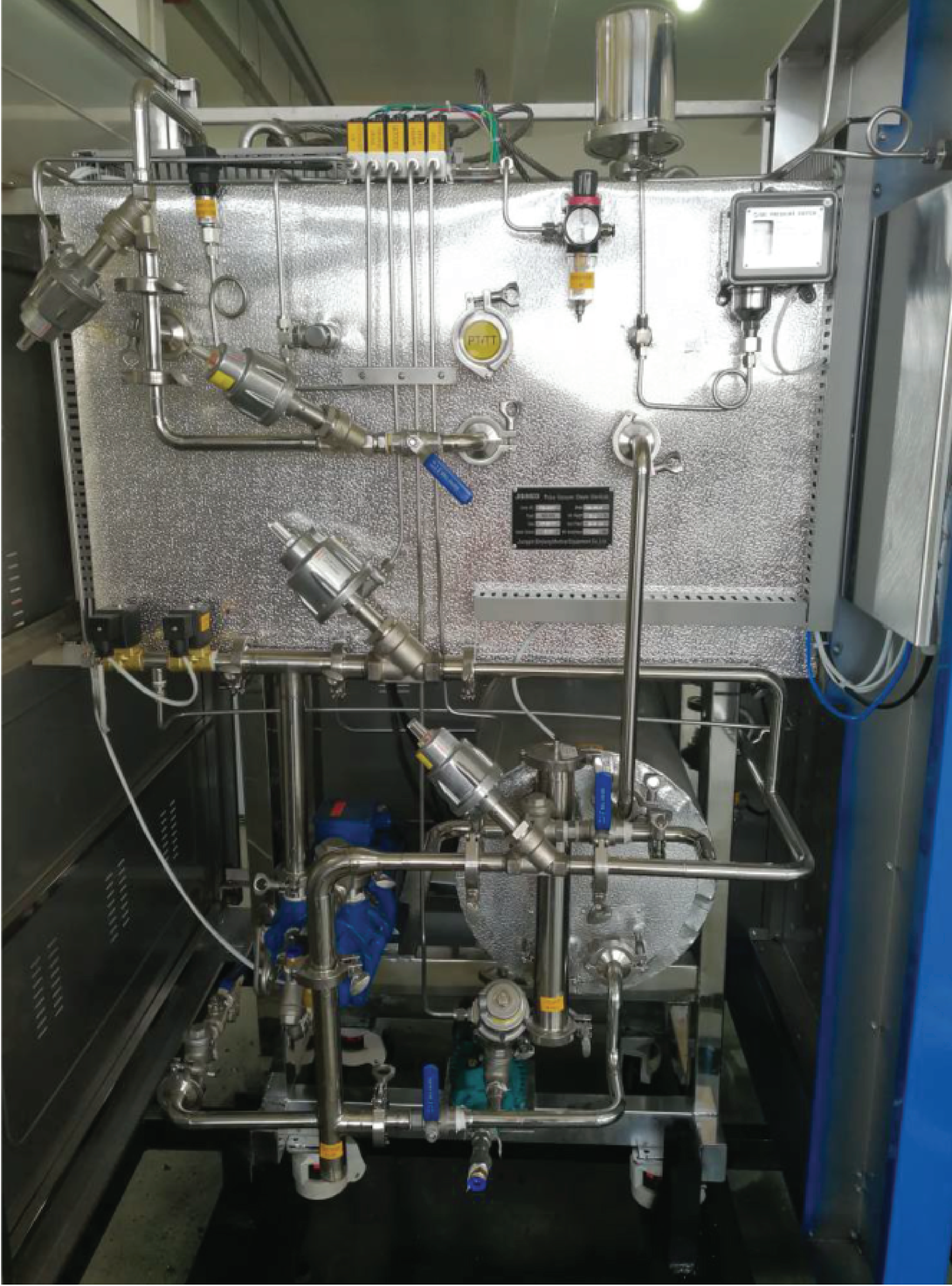
A: Compressor System with connections
